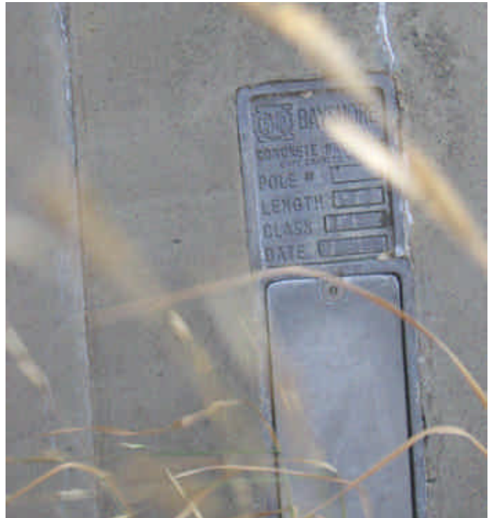
Figure 3 - D Vertical crack from top right of hand hole. Efflorescence buildup is present.
