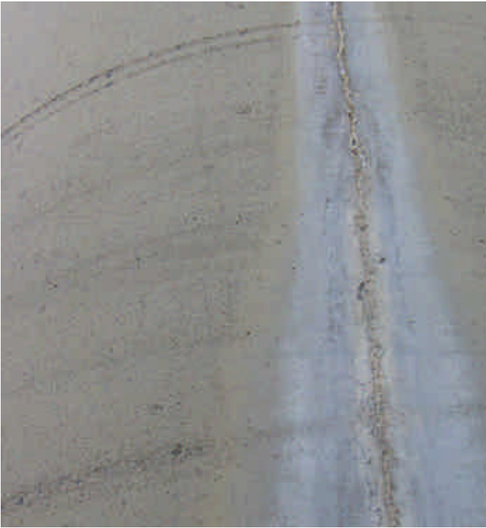
Figure 3 - A A shallow vertical crack at production formwork edge.
