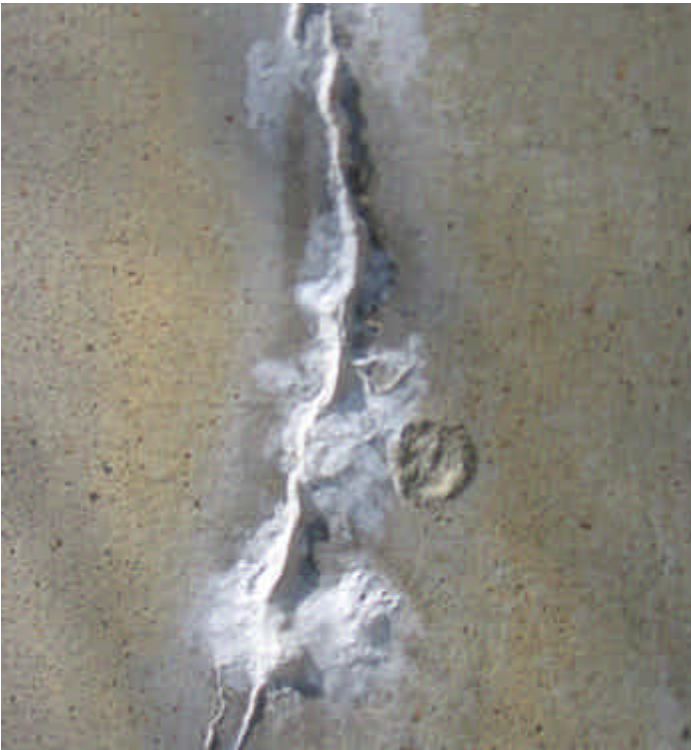
Figure 6 - C Shallow vertical crack with efflorescence buildup.
