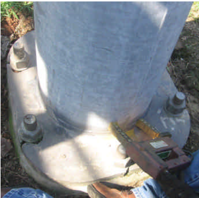
Figure 4 - C A non-destructive Magnetic Particle (MP) test. All four poles were tested.
