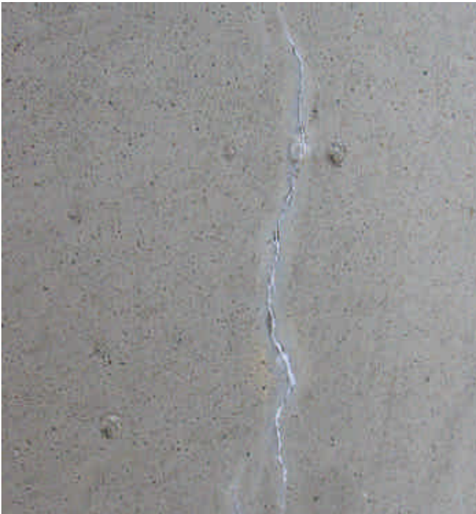
Figure 2 - C Vertical crack with efflorescence buildup.
