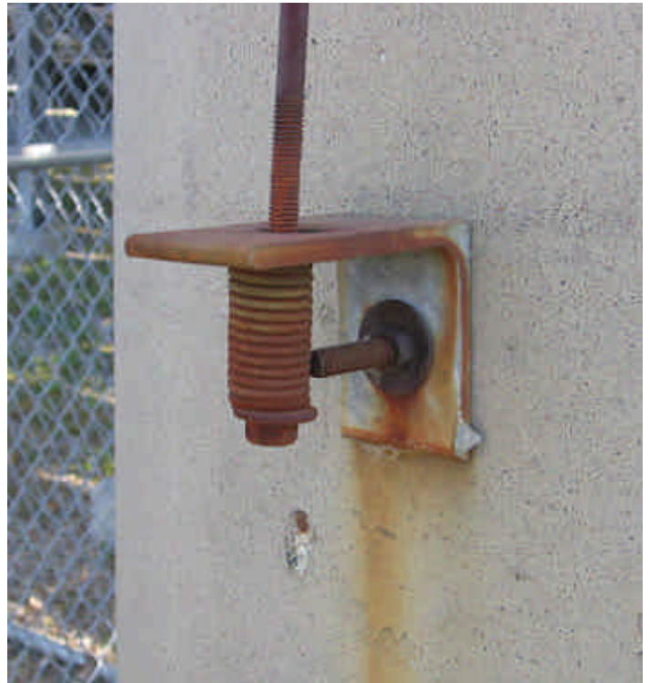
Figure 2 - D Rusted support for the safety cable.
