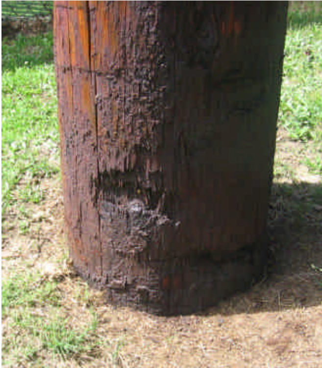
Figure 8 - A Some section loss on two sides of the pole.
