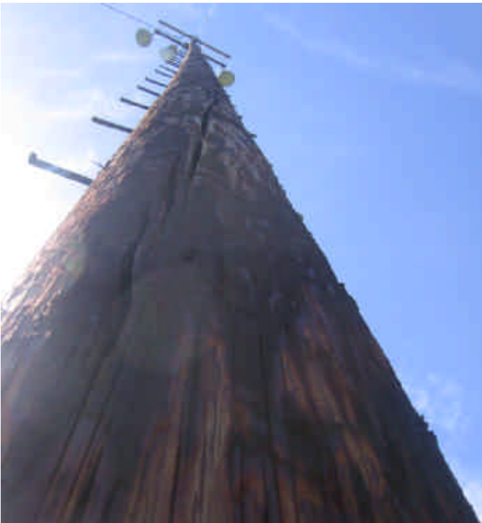
Figure 9 - C Vertical checks near mid height of pole.
