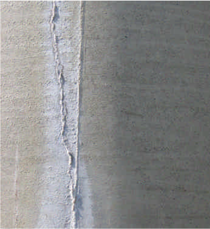
Figure 6 - A Vertical crack with efflorescence buildup.
