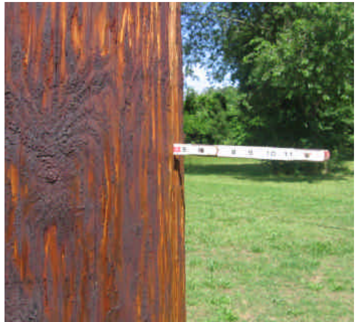
Figure 7 - B Vertical 5"+ check in wood pole. Checks are splits that cross the growth rings.
