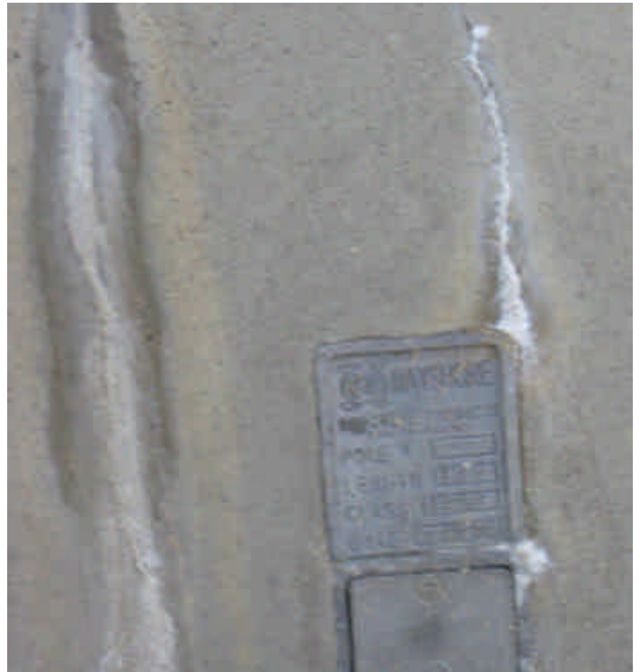
Figure 4 - D Vertical crack from top corner of hand hole with extensive efflorescence.
