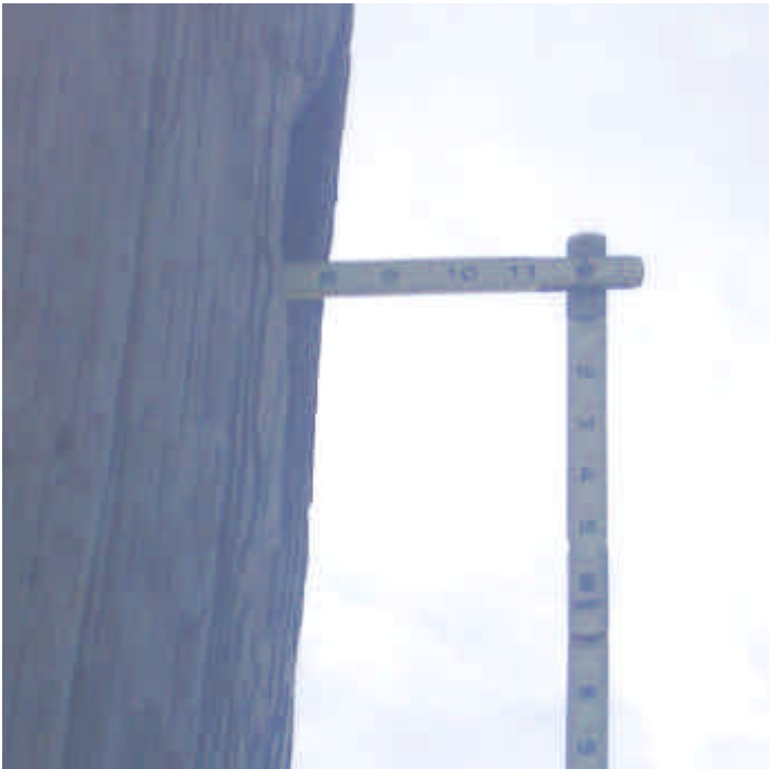
Figure 7 - A Deep hole (8" +) in side of pole large enough to hold a bird.
