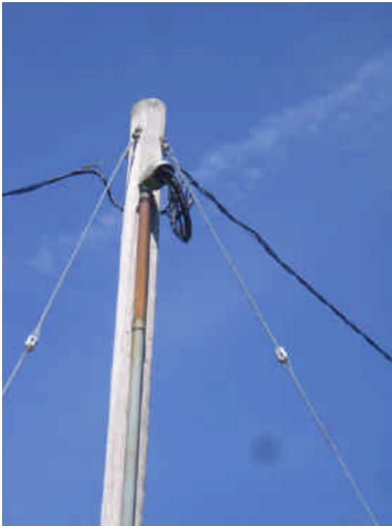
Figure 6 - A Pole with electrical,etc. wires that lead to light poles. Pole not included in contract.
