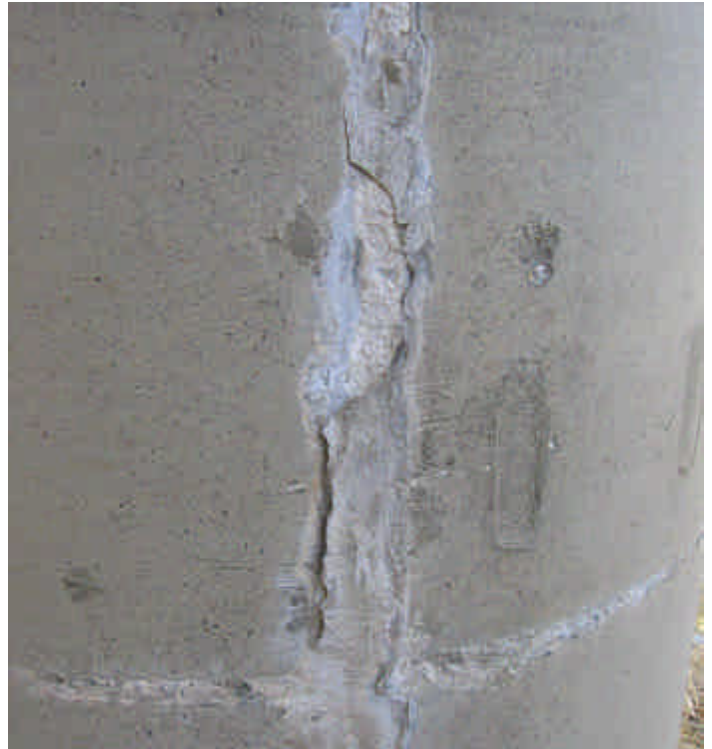
Figure 2 - B A vertical crack with deteriorated repair material.
