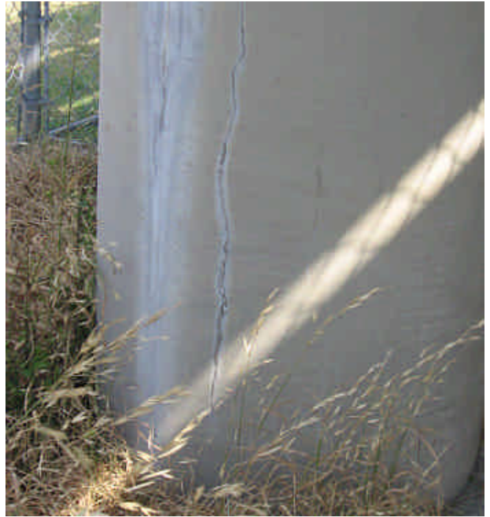
Figure 3 - B Two vertical cracks, one at formwork edge and one parallel.
