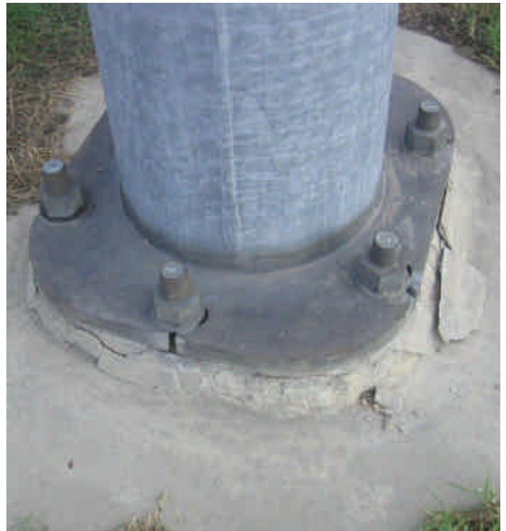
Figure 3 - D Spalled and cracked grout pad.
