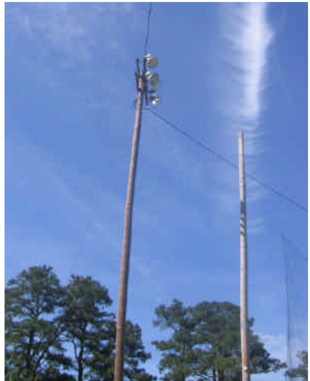
Figure 8 - D Typical pole with out-of-plumb variations over total height.
