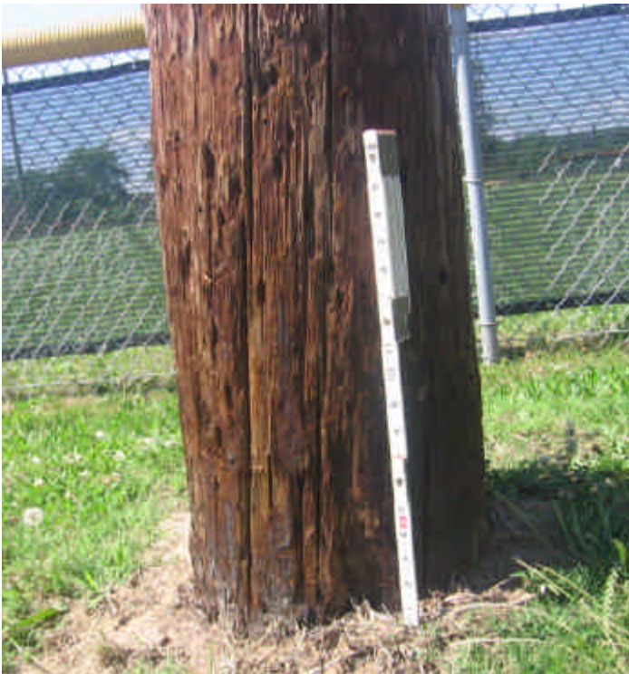
Figure 7 - C Vertical checks. Moisture and incising treatment is indicated by the small holes.
