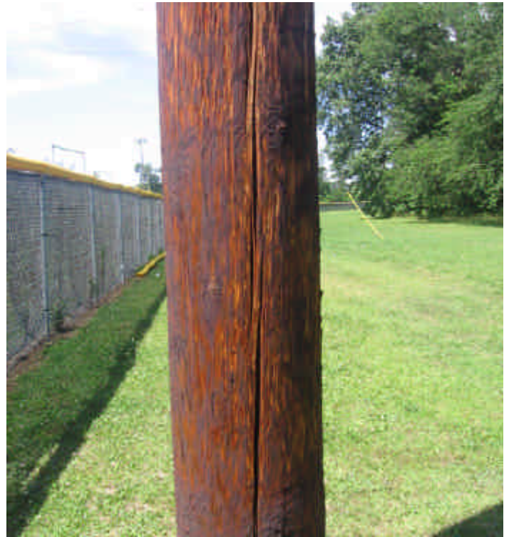
Figure 9 - B Vertical checks. Tar moisture treatment is visible at the base.
