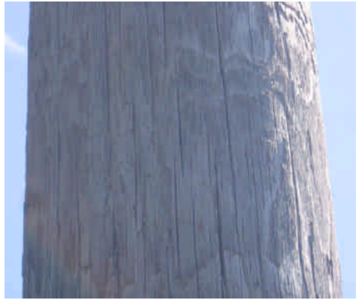
Figure 8 - B Typical small surface checks.
