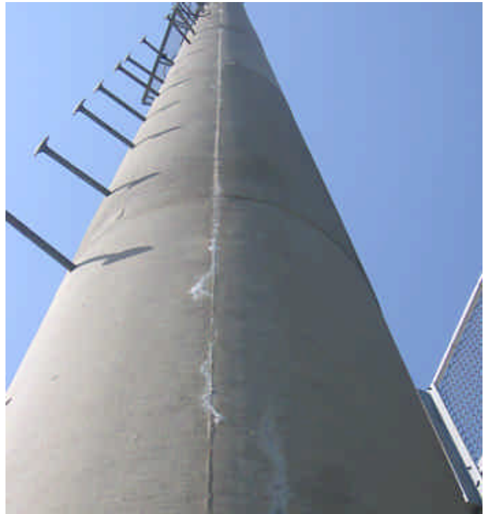
Figure 5 - D Efflorescence buildup at vertical crack in pole 2.
