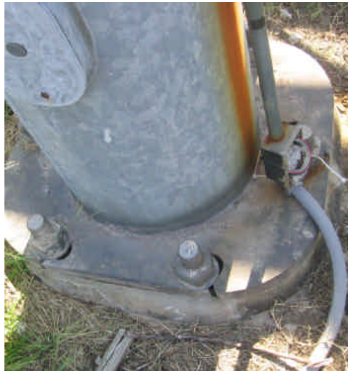
Figure 1 - D Rust stains near conduit attached to the light pole.
