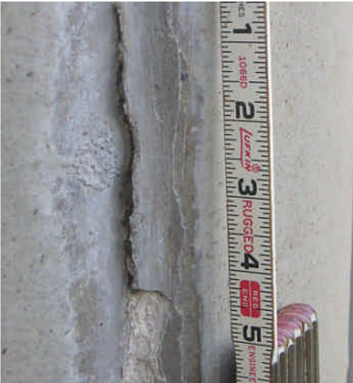
Figure 4 - C Loose repair material at formwork edge.
