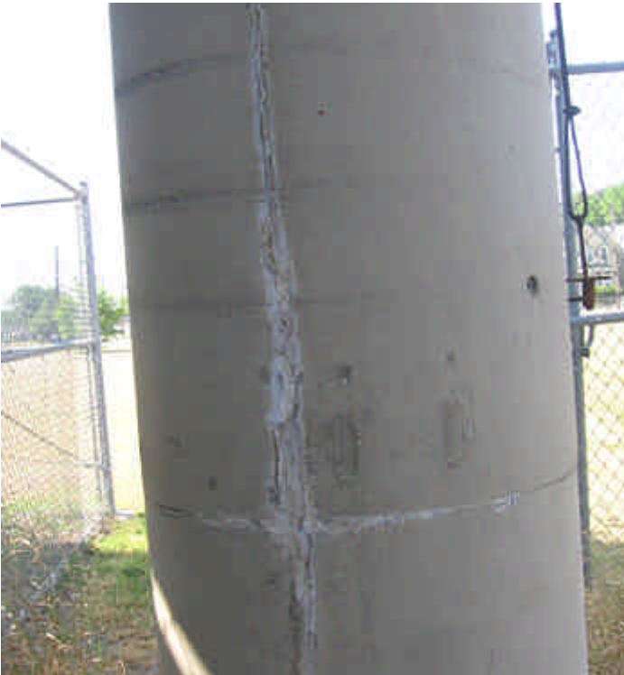
Figure 3 - C A shallow vertical crack at formwork edge on pole 4.
