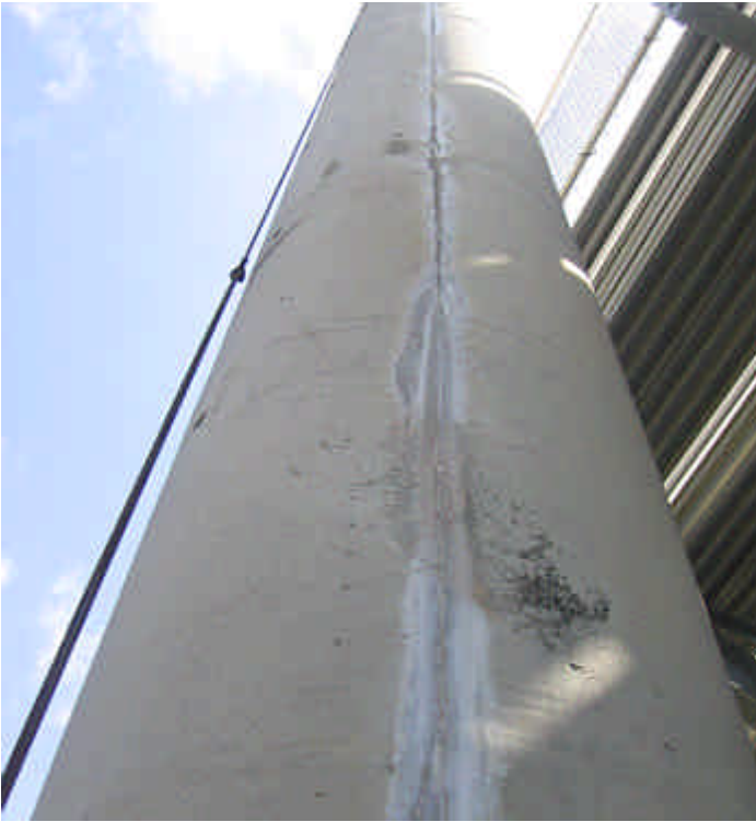
Figure 4 - A An extensive shallow vertical crack at formwork edge.
