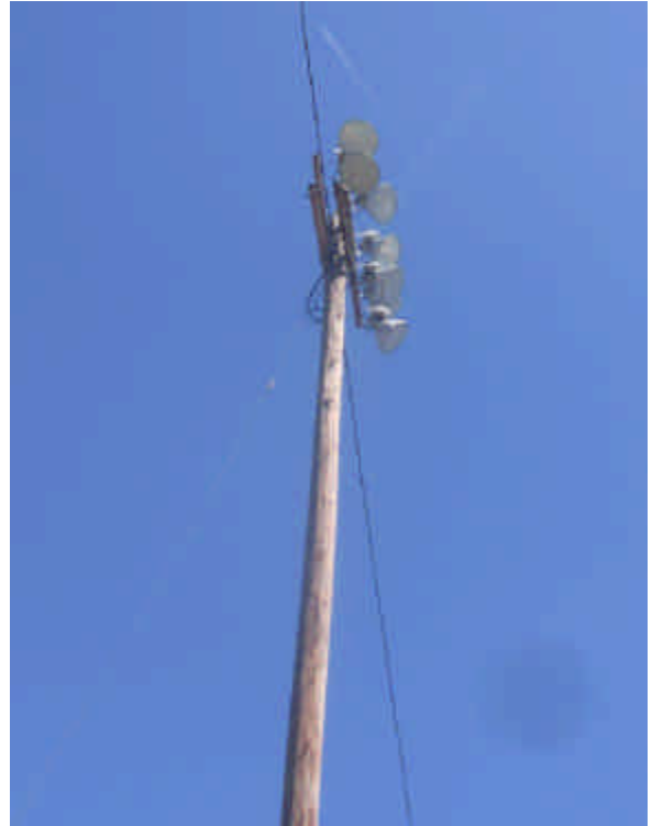
Figure 5 - B Typical light package at the top of the wood baseball poles.
