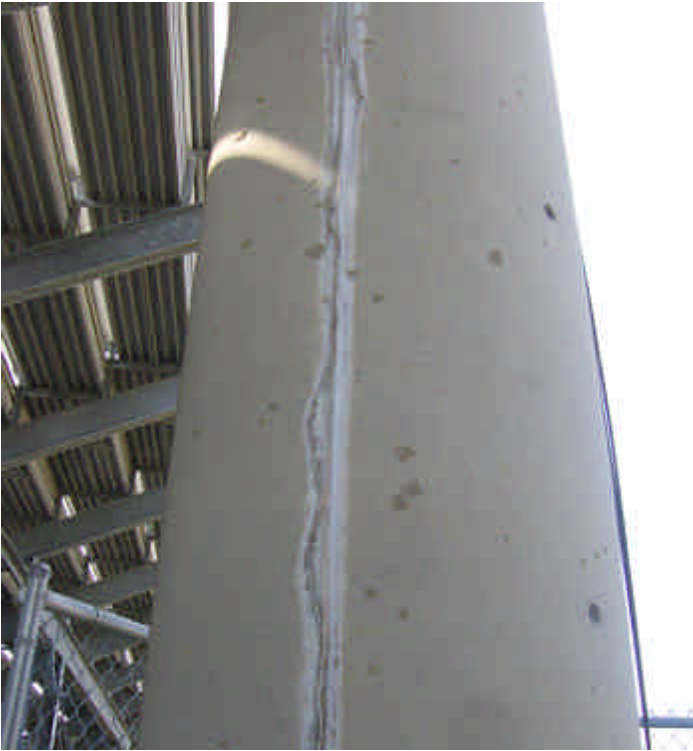
Figure 5 - A Tall vertical crack at pole 3.
