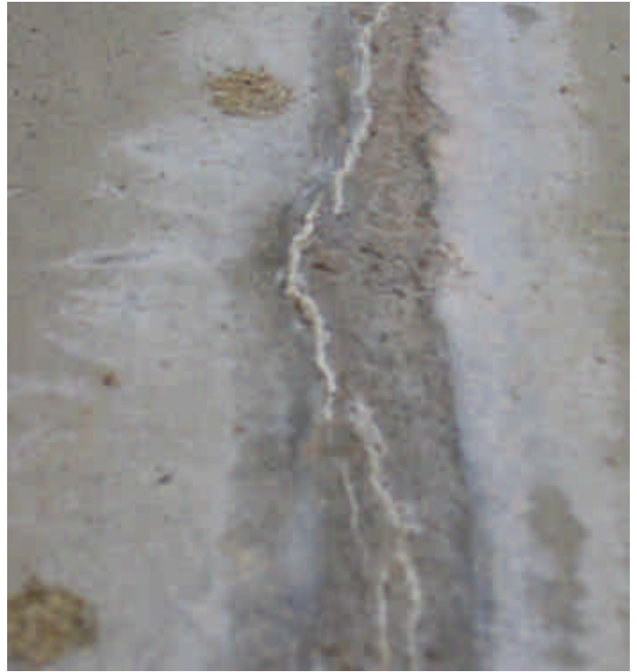
Figure 4 - B Shallow vertical crack with missing repair material.
