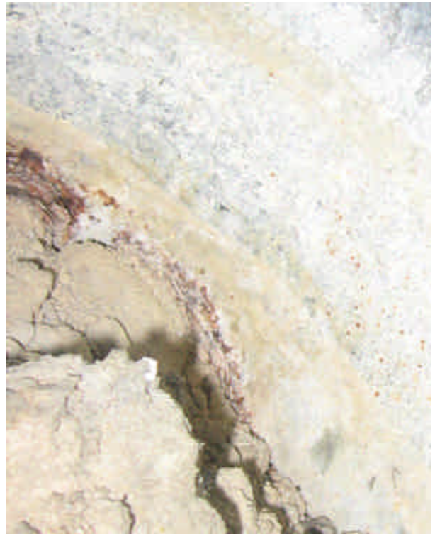
Figure 4 - B Potential rust or rust stains inside the pole at the base plate.
