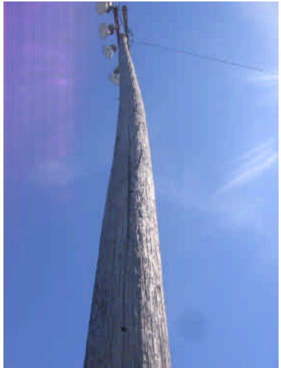
Figure 6 - B Lightpole with noticable out-of-plumb change near mid height.
