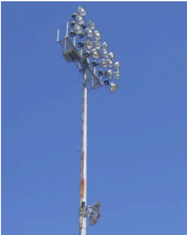
Figure 1 - C A football lightpole with speakers. Rust stains are seen on side near conduit.
