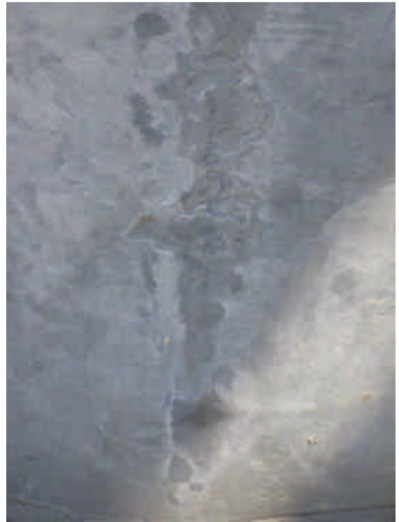
Figure 3 - B Surface damage to galvanizing layer.
