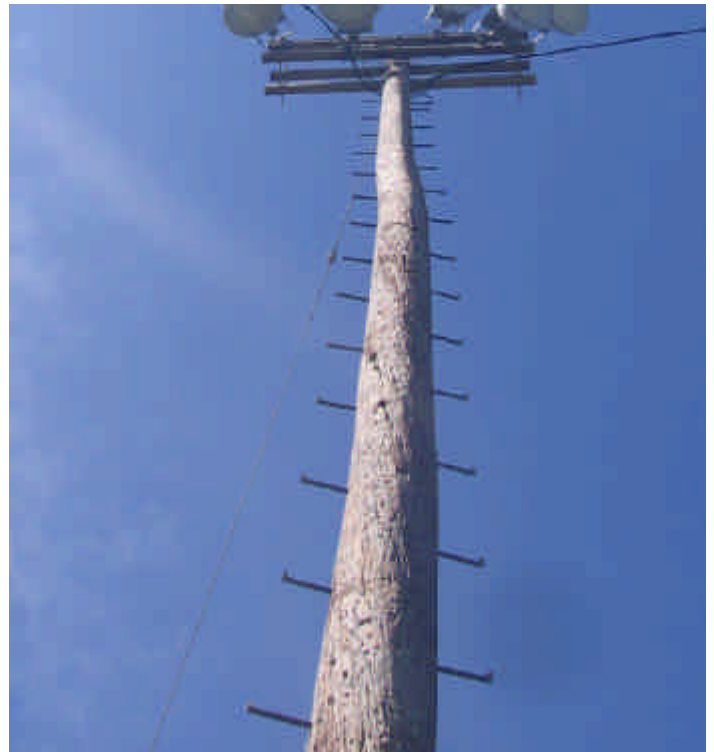
Figure 9 - D Distinct out-of-plumb transition near top of pole.
