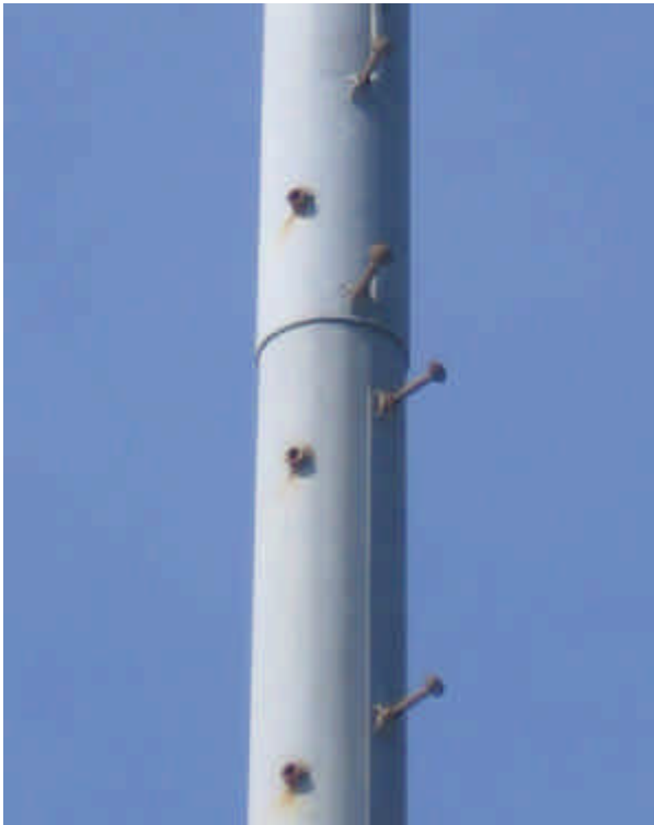
Figure 4 - A Potential rust or rust stains mid height of pole near hand holds.
