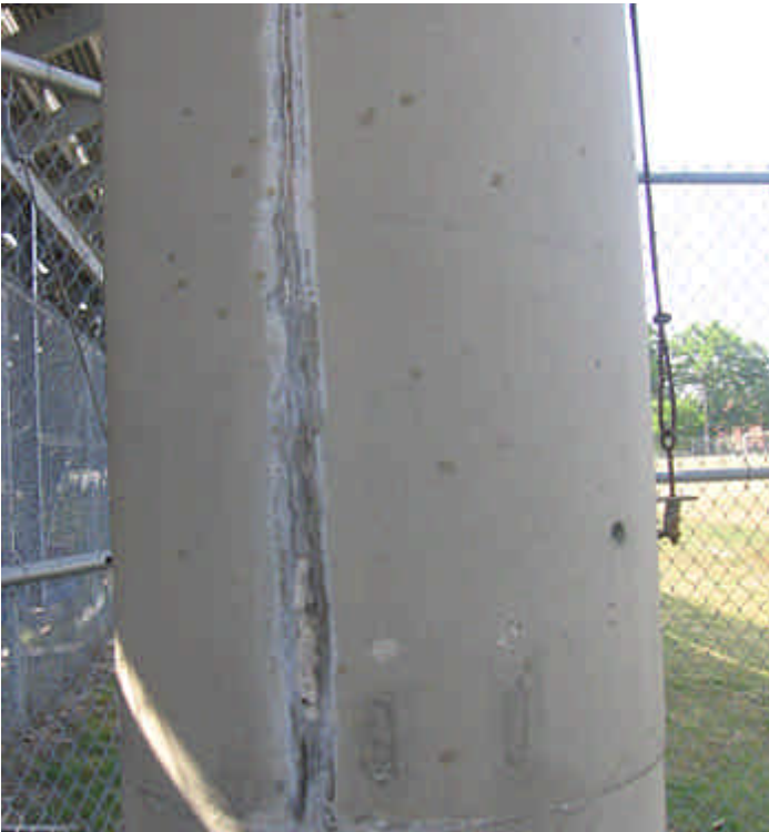
Figure 5 - C Lower portion of vertical crack at pole 3. Repair material is loose.
