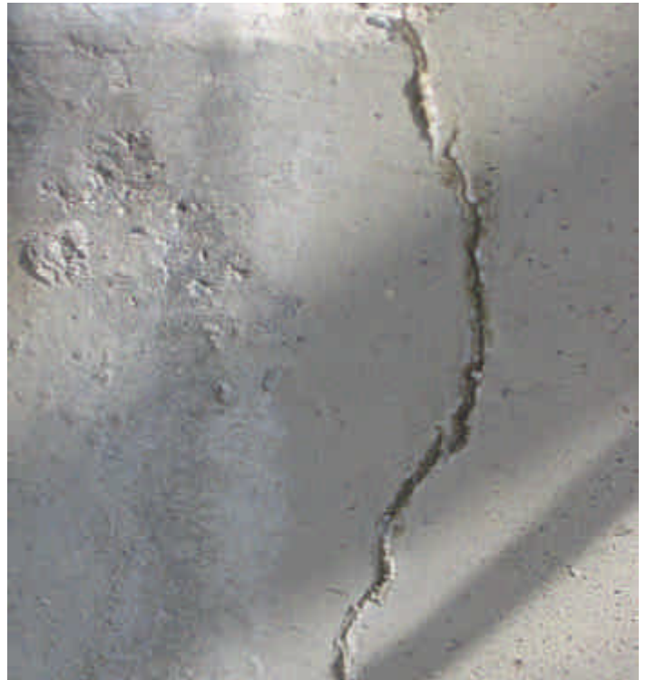
Figure 6 - D Vertical crack from bottom right corner of hand hole.
