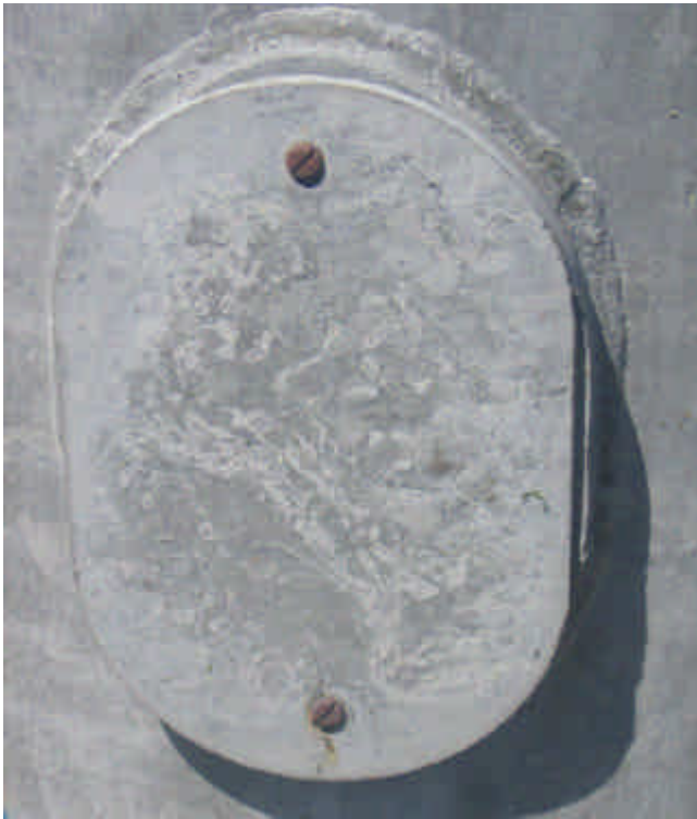
Figure 3 - A Typical hand hole on the light poles.
