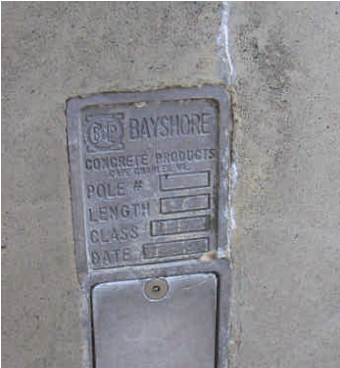
Figure 2 - A A vertical crack occurring at the top right of the hand hole.
