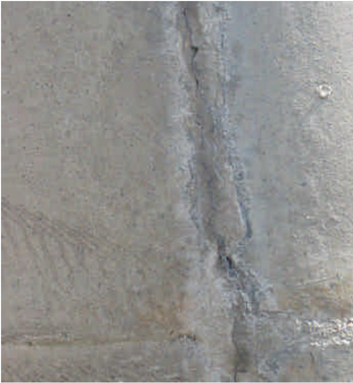
Figure 7 - A Vertical crack with some repair material missing.
