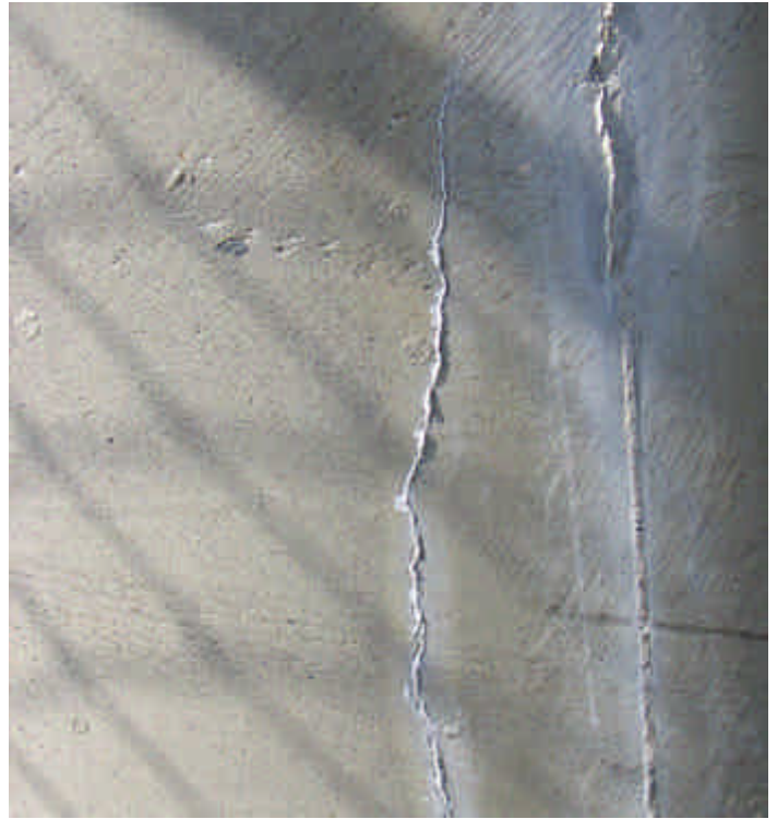
Figure 6 - B Vertical cracks at panel edge and parallel with efflorescence buildup.
