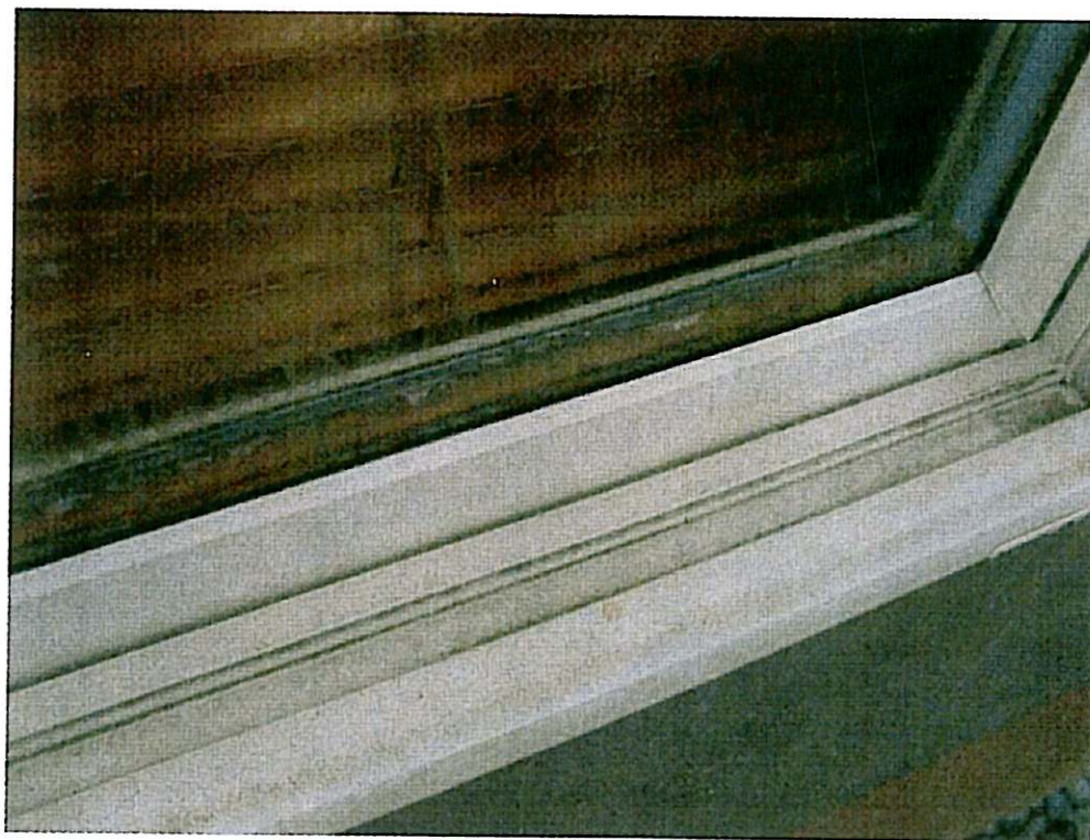
Figure 4. Failed double-pane window
