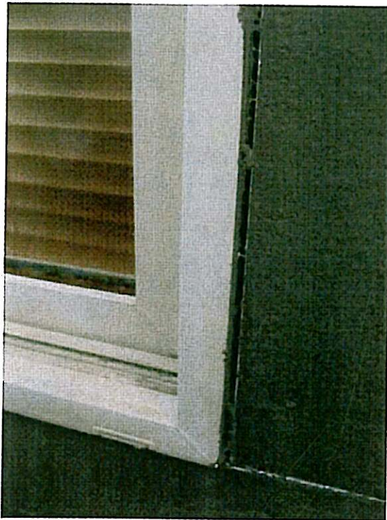
Figure 5. Window separating from siding
