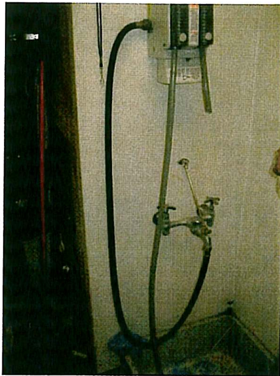
Figure 9. Custodian's hot/cold water faucet
