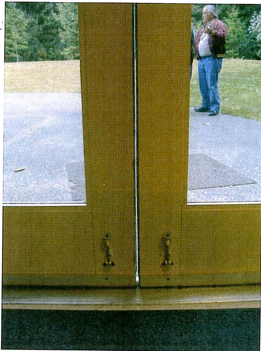
Figure 2. Gap in closed exterior doorway
