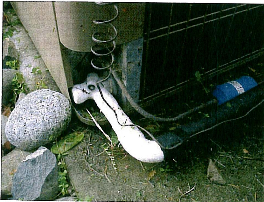
Figure 8. Iced-up refrigerant line on air conditioner
