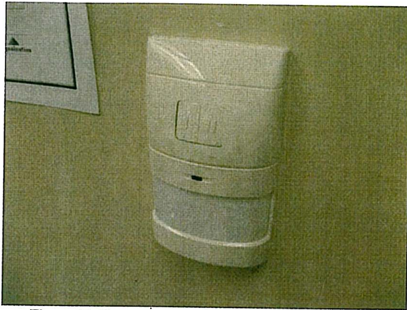
Figure 11. Occupancy sensing two-level light switches
