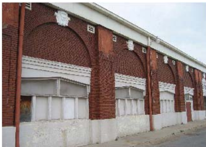
Figure 6 —Detail photo of West Façade. Note repetitive façade details including brick masonry arch, architectural concrete keystone, brick masonry pilasters, concrete flat arches/beams. Also note removed medallions at pilasters and removed cornice at roof edge now wrapped in Mapes panels. Photo - D.Worth and S. Kelley Sept 2009
