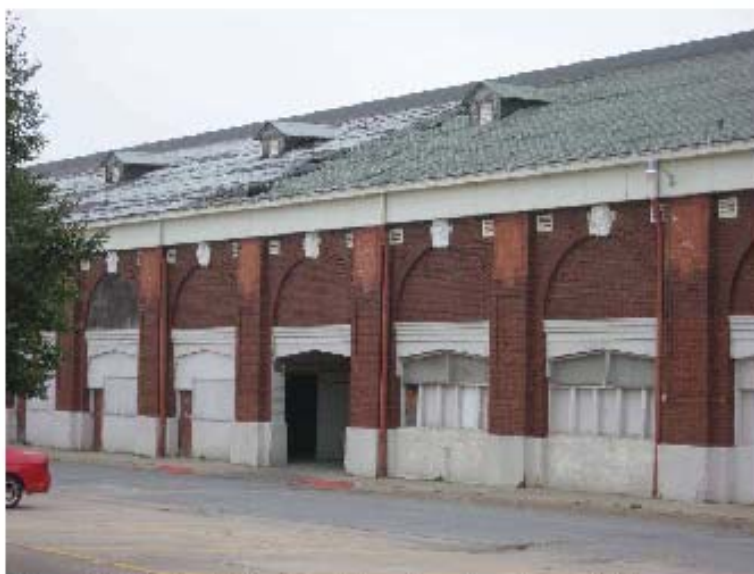
Figure 9 —Photo detail of west façade and roof area. Note deteriorated roof coverings and dormers modified with mechanical louvers and fans. Photo - D.Worth and S. Kelley Sept 2009
