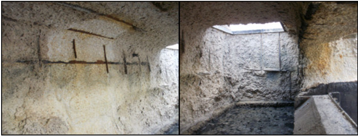
Photo 14 (left): Exposed and corroded reinforcement in the wall section hydro-blasted by the Contractor.
