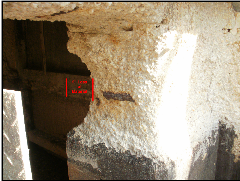
Photo 2: Chemical attack and corroded reinforcement of west wall at the northwest corner of the grit chamber. Note the wall is common to the influent channel beyond.
