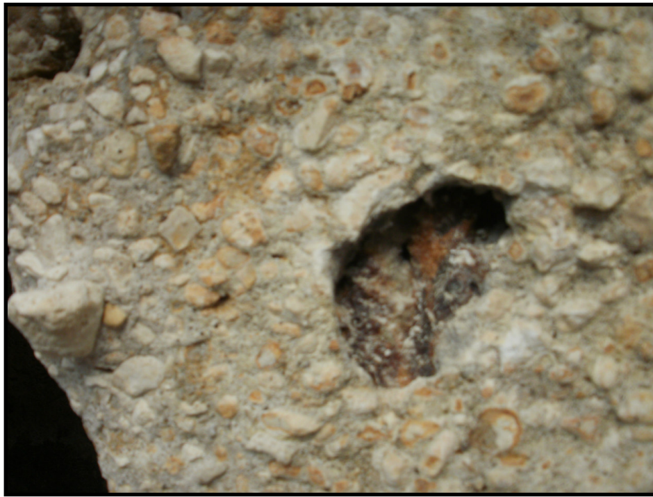
Photo 8: Close-up view of corroded reinforcement within the void.
