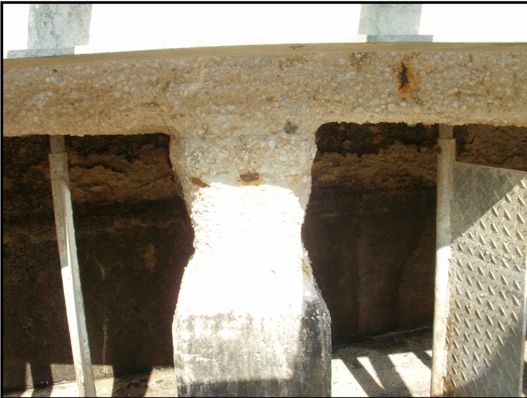
Photo 4: Chemical attack and exposed and corroded reinforcement of west wall at the support section of concrete at the approximate center of the opening to the influent channel beyond.
