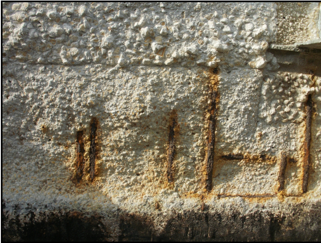
Photo 3: Chemical attack and exposed and corroded reinforcement at the south wall.
