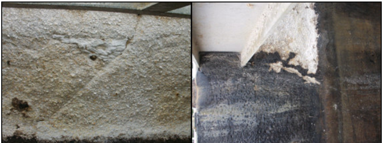
Photos 9 and 10: Diagonal cracks observed in the north wall at aluminum beam embedment locations.
