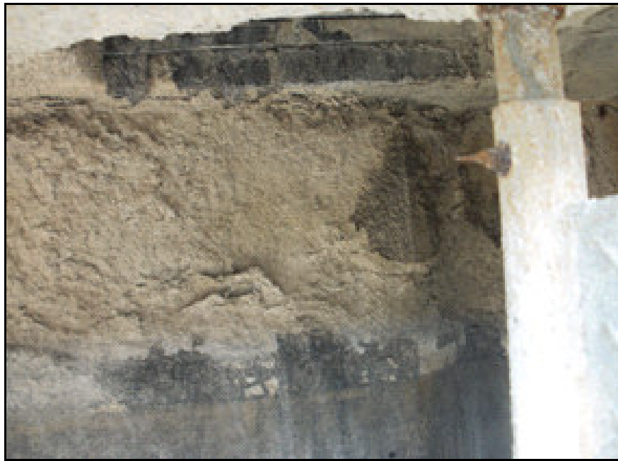
Photo 13: Condition of the influent channel west wall, typical of channel walls observed during our review.
