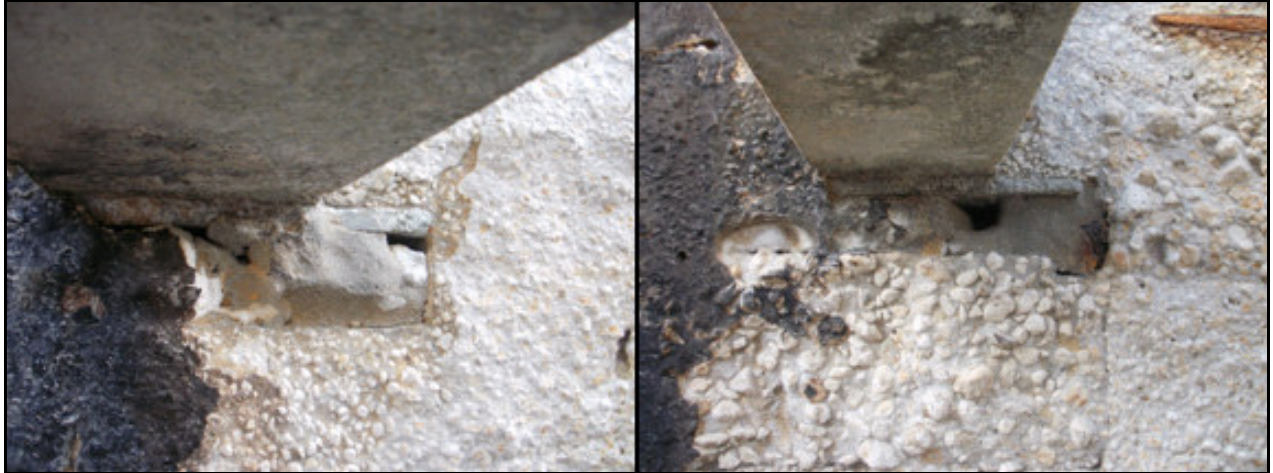
Photos 11 and 12: Deterioration of grout and voids at embedment locations of aluminum beams.
