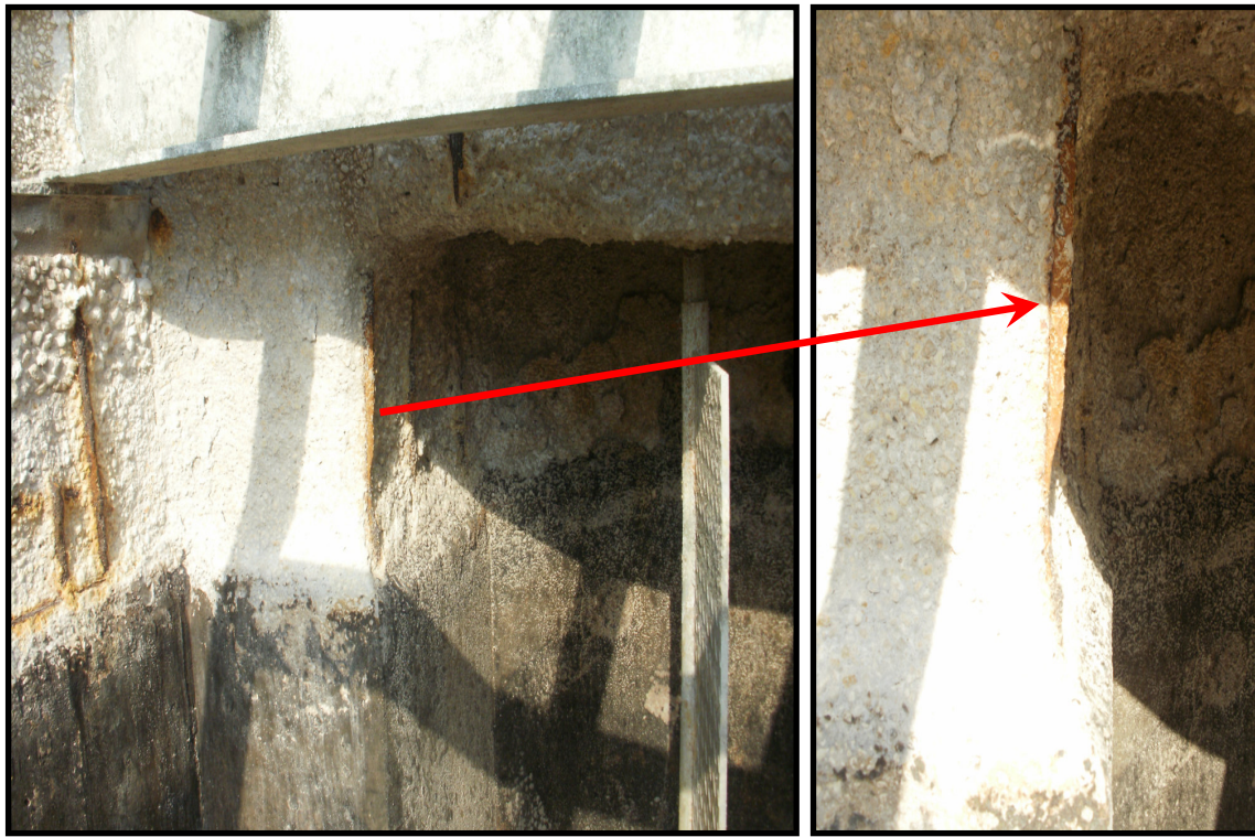
Photos 5 and 6: Exposed and corroded reinforcement of the west wall at the southwest corner of the grit chamber. Note the wall is common to the influent channel beyond.
