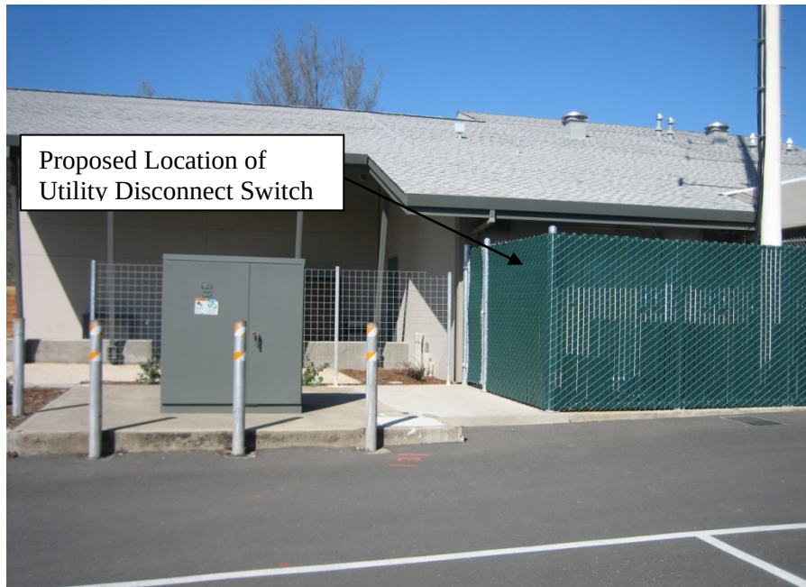
Photo 3 – Proposed Location of Utility Tie-In and Disconnect Switch
