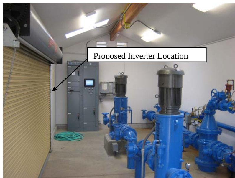
Image 12 - Pump Station Inverter Location
