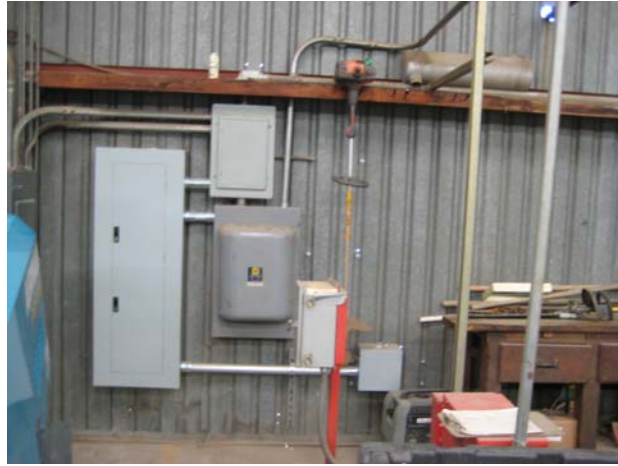
Image 3 - Corporation Yard Warehouse Bldg. Inverter Location
