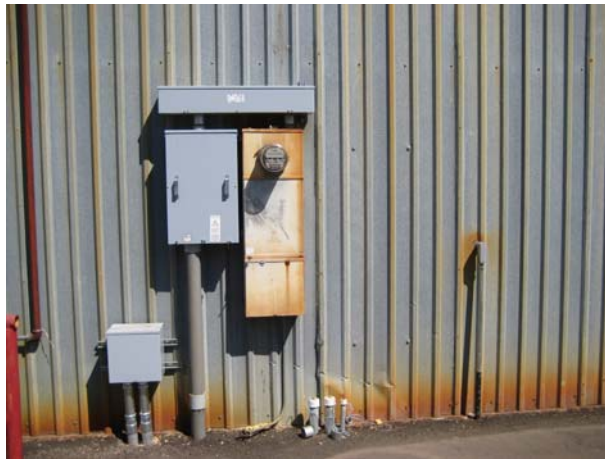
Image 1 - Corporation Yard PG&E Service Meter
