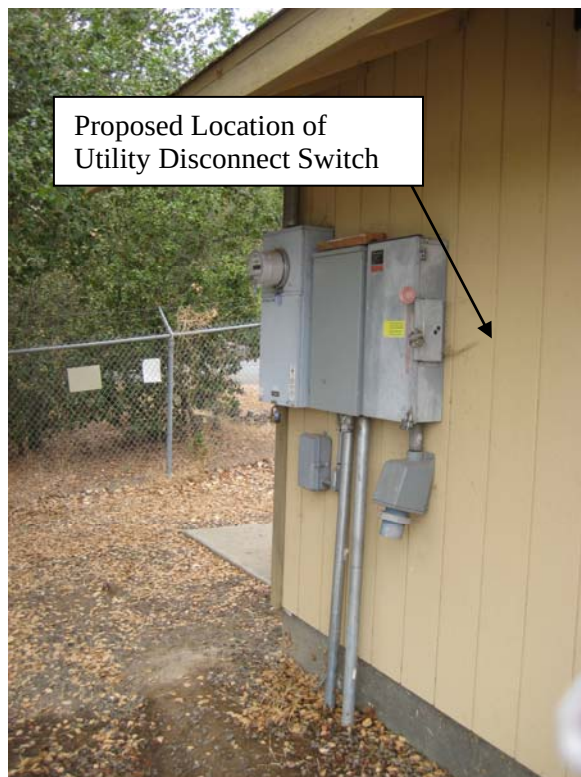
Image 13 - Pump Station Utility Disconnect Switch Location
