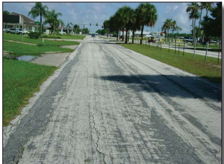
Photo 12 Existing pavement is in poor condition north of Franklin Drive on Clearmont Street.
