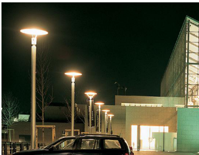
Indirect parking lot lighting
