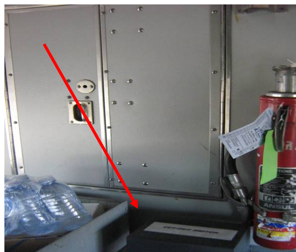
PTC Cut-Out switch Cab Cars (4021-4026)
