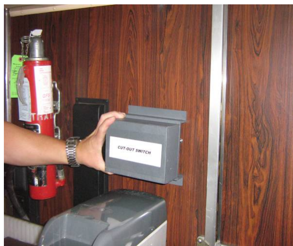
PTC Cut - Out Switch Cab Cars (Cars 4000-4020)
