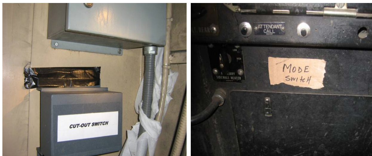
Figure 9 - Potential Location for PTC Activation Switches - EMD F40PH-2
