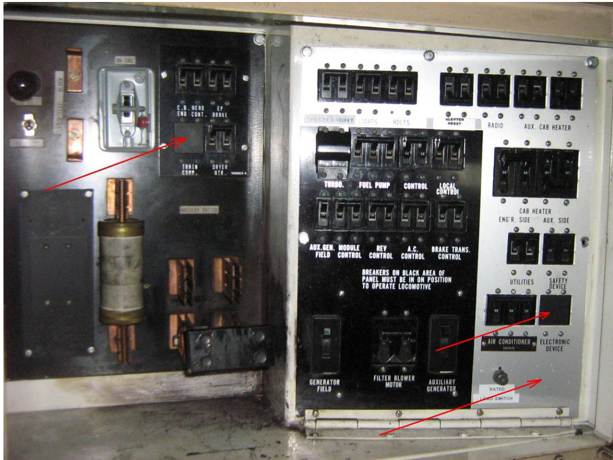
Figure 6 - Circuit Breaker Panel EMD F40PH-2
