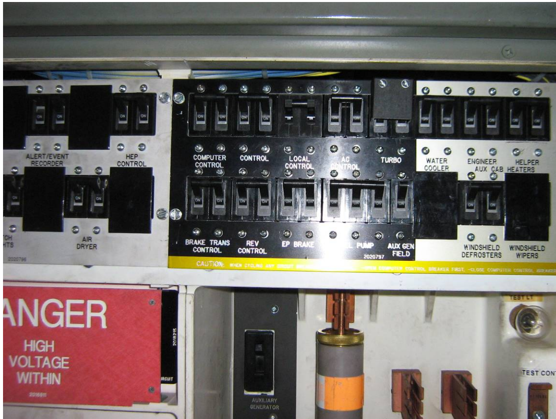
Figure 16 - MP36 Circuit Breaker Panel
