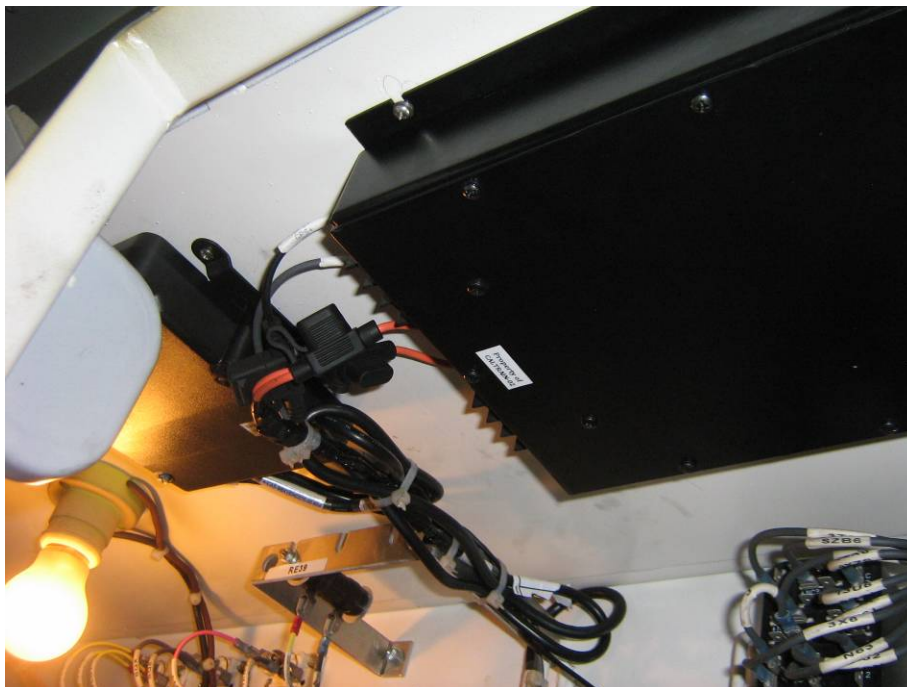
Figure 17 - Installed AVL Equipment - MP36
