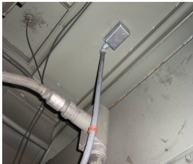
GPS Antenna Junction Box
