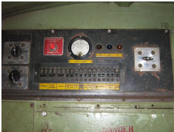
GP9 Circuit Breaker Panel
