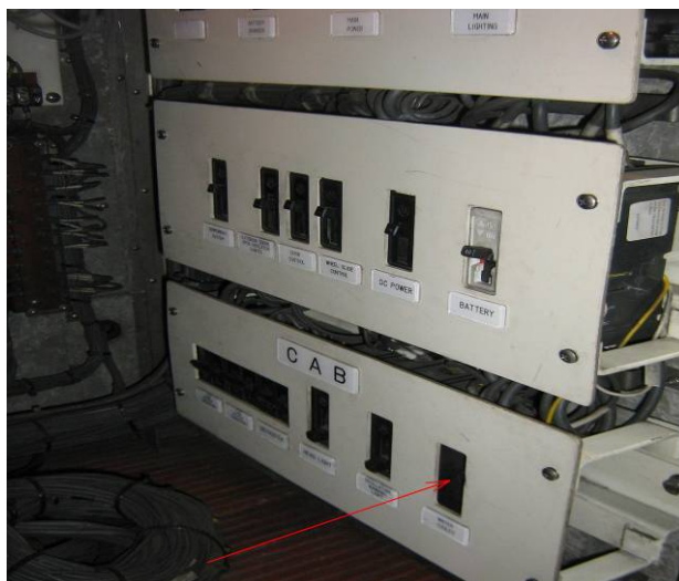
Breaker Panel (Cars 4000-4020)
