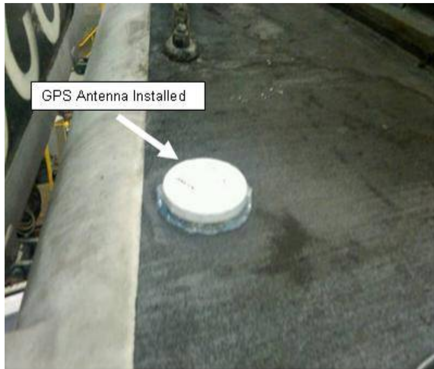
Figure 11 - AVL Equipment Installed
