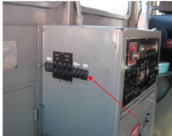
MP15 Circuit Breaker Panel
