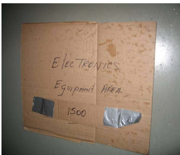
MP15 Equipment Enclosure Area
