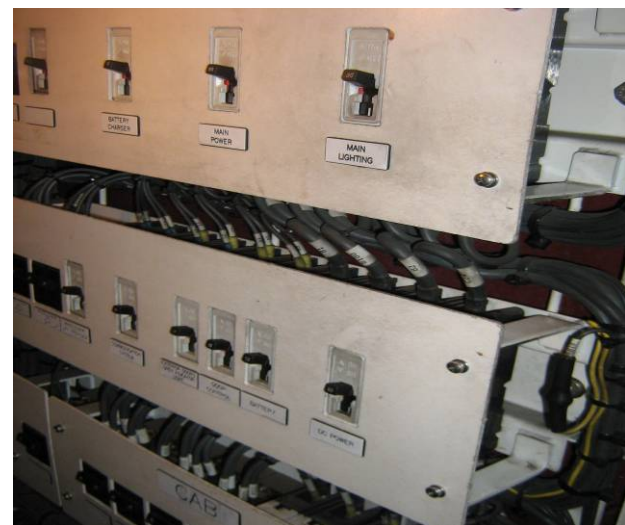
Breaker Panel (Cars 4021-4026)
