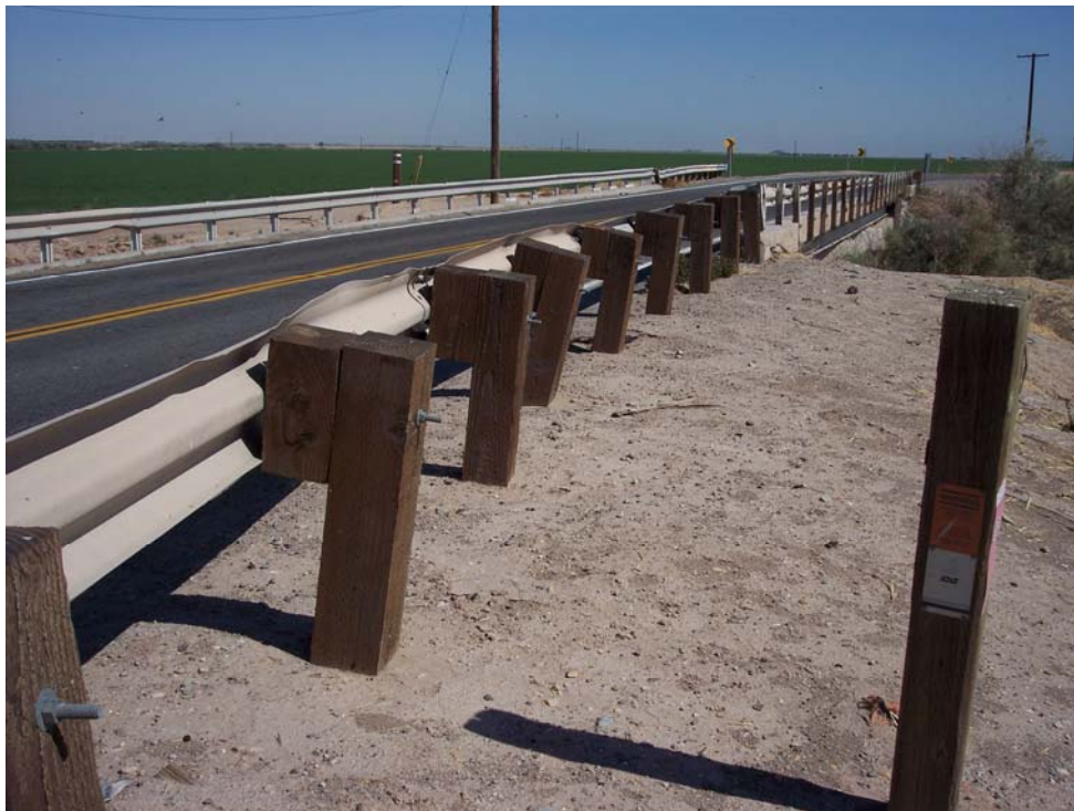
Figure 2: Northbound Approach and Guard Rail Facing Northwest June 19, 2008
