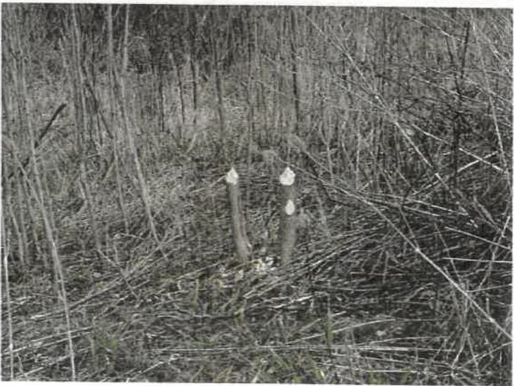
9. A view of rodent activity on the downstream slope.
