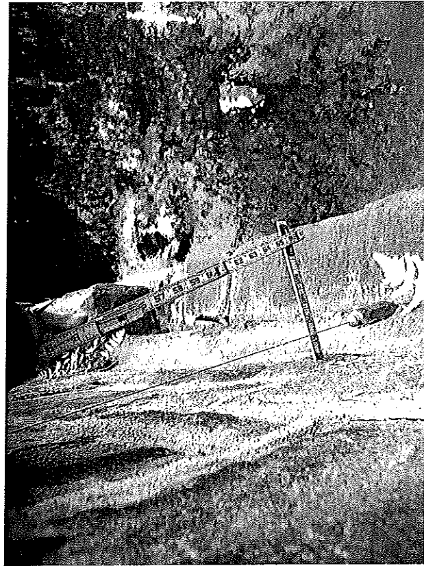
Photo # 12: Tipping of the north parapet.
