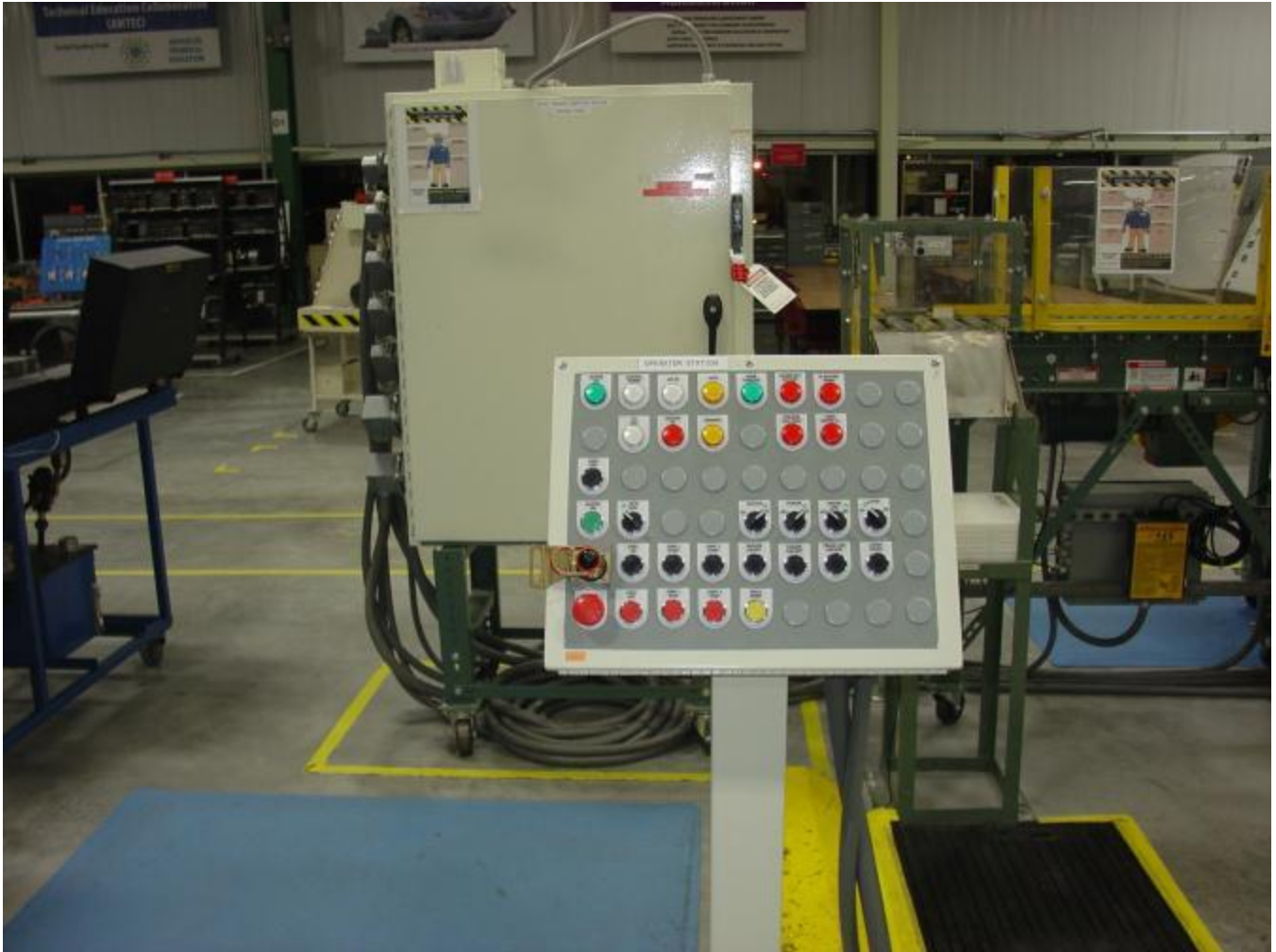
Operator Control Panel
