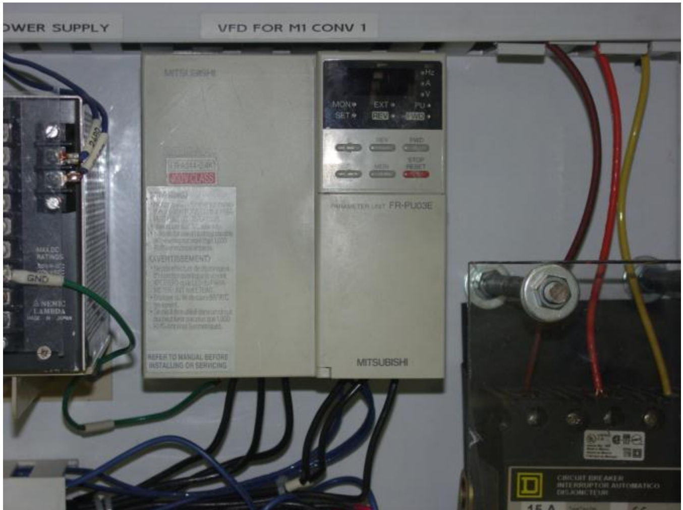
Cabinet Interior – Inverter
