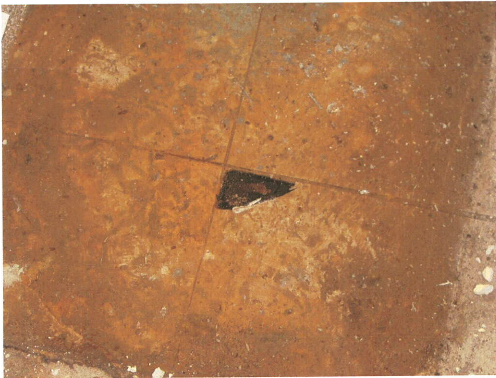
Photo 6: Typical ACM Tan VFT with ACM black mastic in some units
