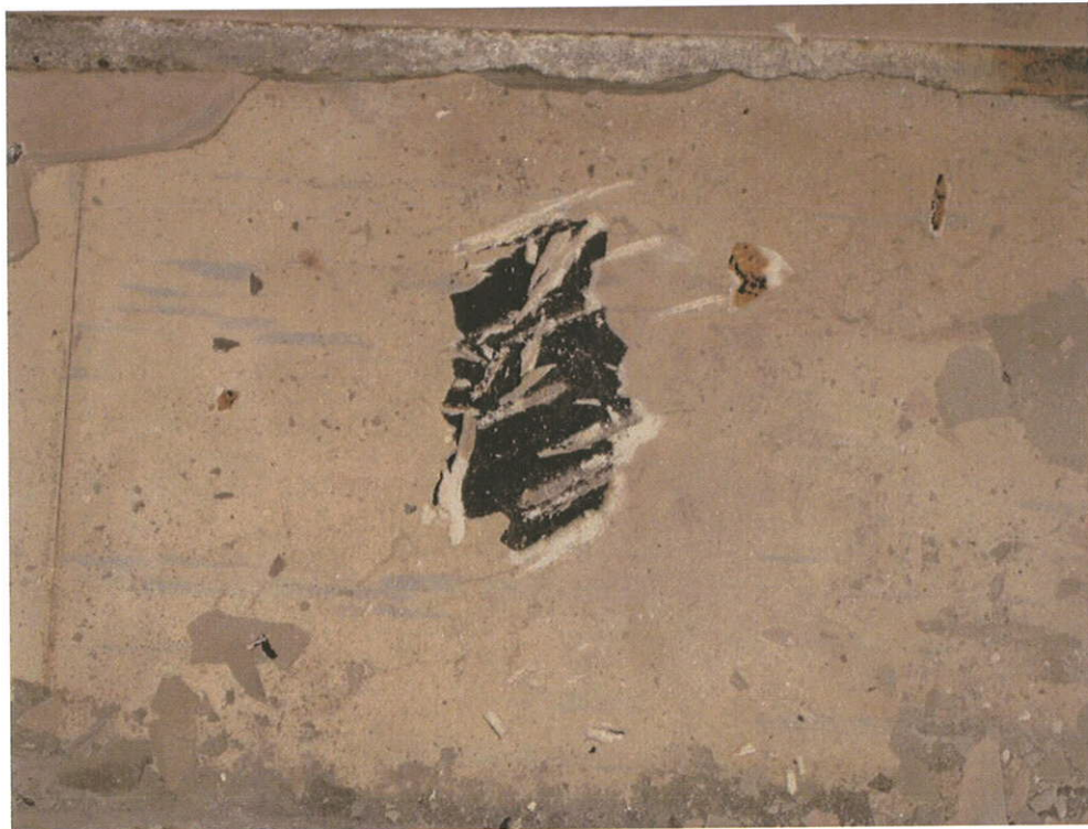
Photo 12: Typical ACM Beige VFT w/black mastic in some units
