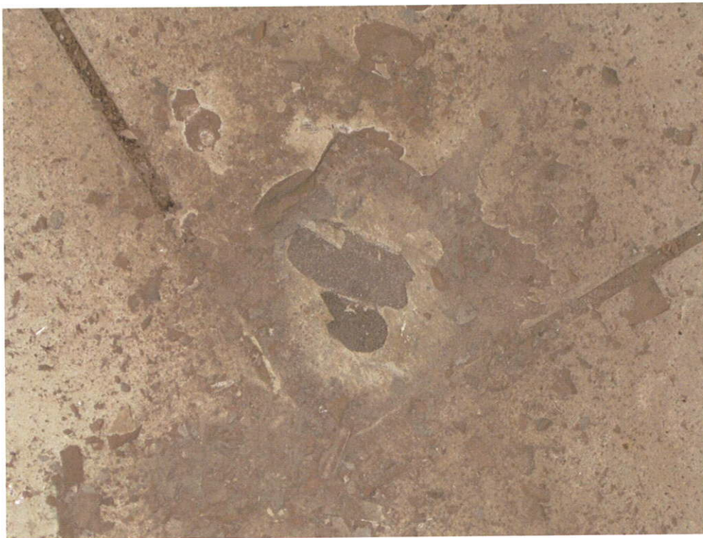
Photo 16: Typical ACM Tan VFT under ceramic tile in some units
