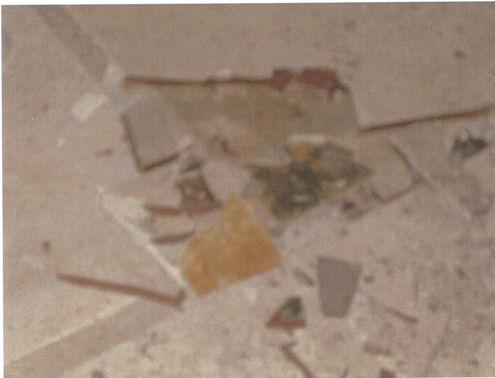
Photo 14: Typical ACM Tan VFT under ceramic tile in some units
