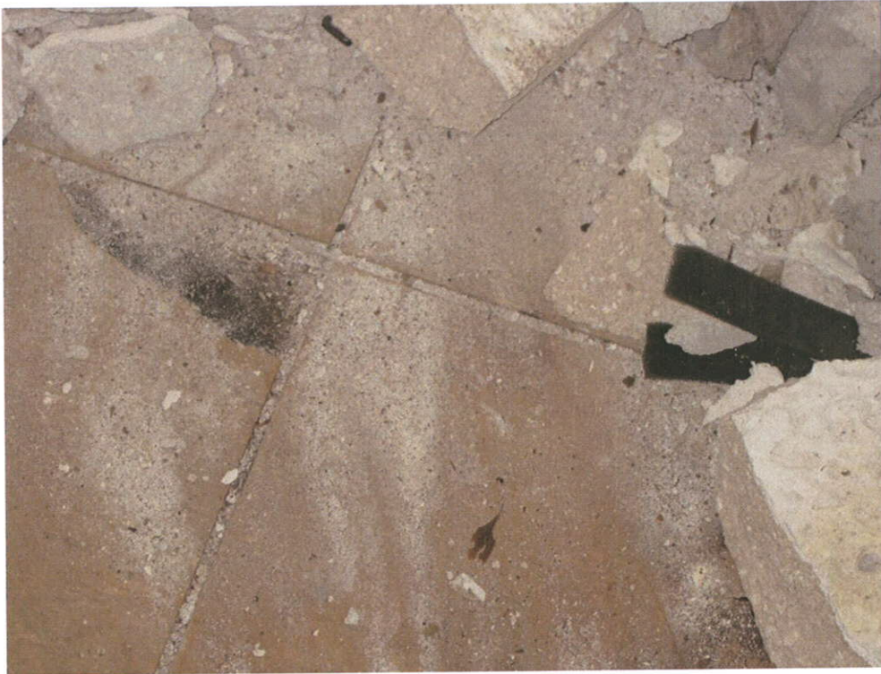
Photo 9: Typical ACM Tan VFT
