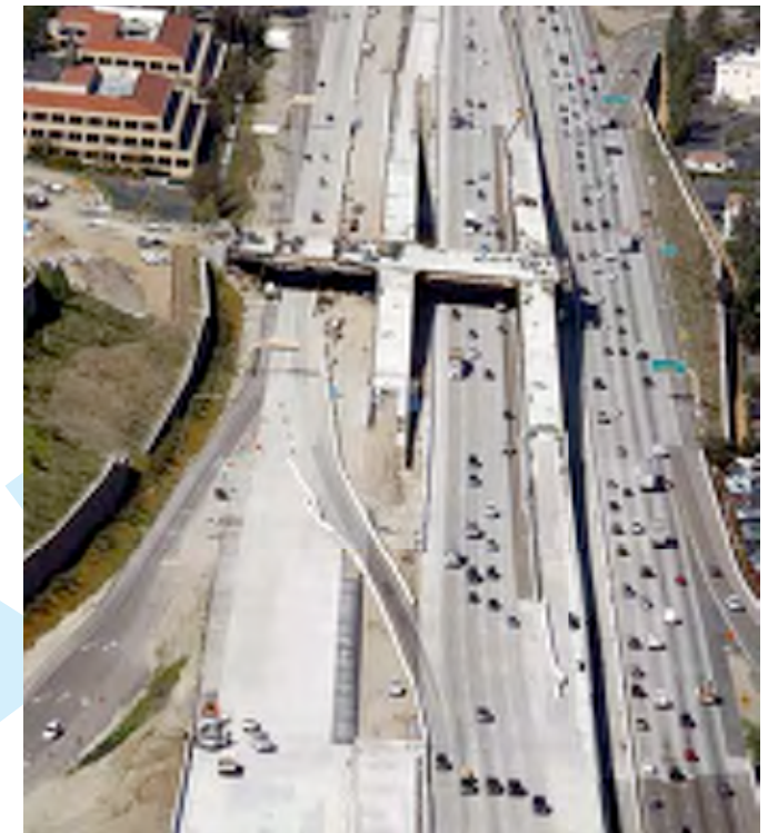
I-15 Construction progress continued with new bridges, expanded lanes, and direct access ramps. In 2008, another 4.5 miles of managed lanes opened from Ted Williams Parkway to Rancho Bernardo Road, extending the existing lanes to 12.5 miles of "expressway-within-a-freeway."
